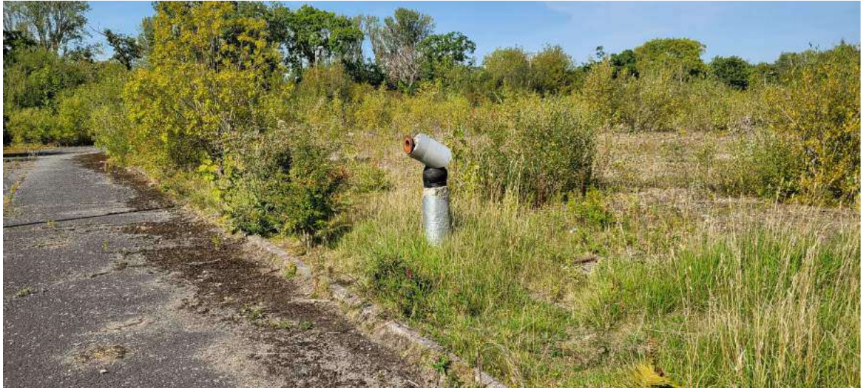
Suspected steam pipe network
