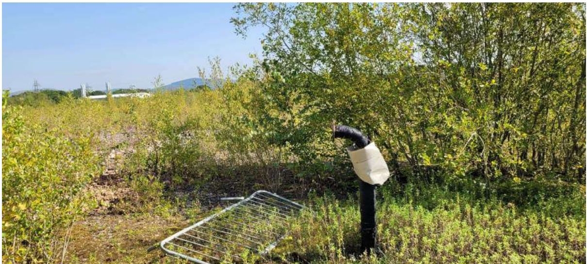
Suspect Steam Pipe Network
